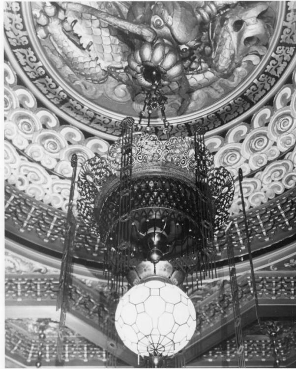
Fig.20 Detail of 5 th Avenue Theater's ceiling light fixture, with emphasis on the "Pearl of Perfection" and Plaster Dragon, 1978 (Washington State Office of Archeology and Historic Preservation)
